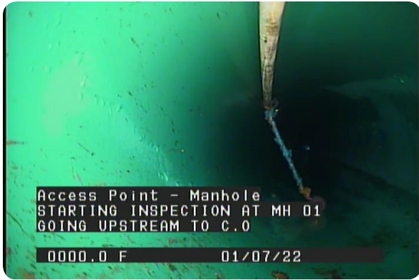
Access Point - Manhole at 000.0 feet | STARTING INSPECTION AT MH 01 GOING UPSTREAM TO CLEAN OUT
